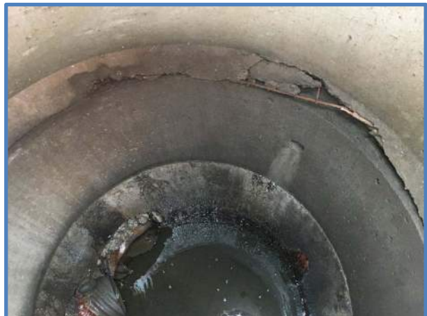
Photo 2 - Cone Damage, Exposed Steel
